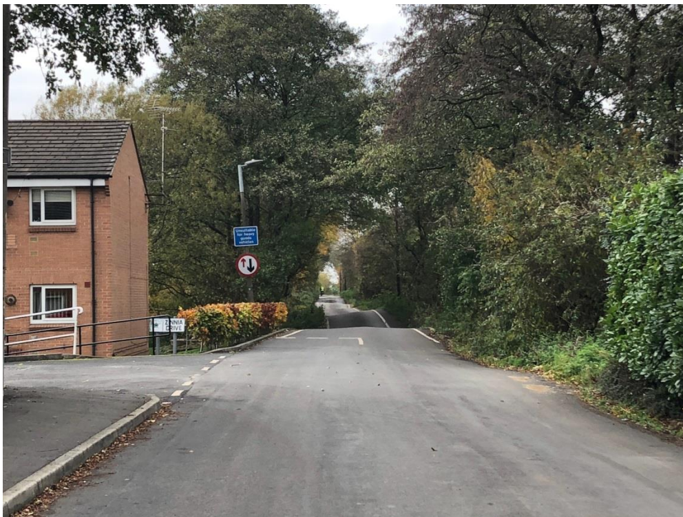
PHOTO 4: VIEW N ALONG ASTLEY ROAD INTO THE SITE (SEVERE SUBSIDENCE OBSERVED)
